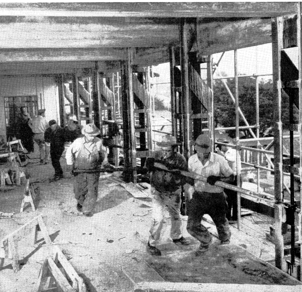
At the long awaited moment, workmen simultaneously started to turn the screws lowering the giant slab.
